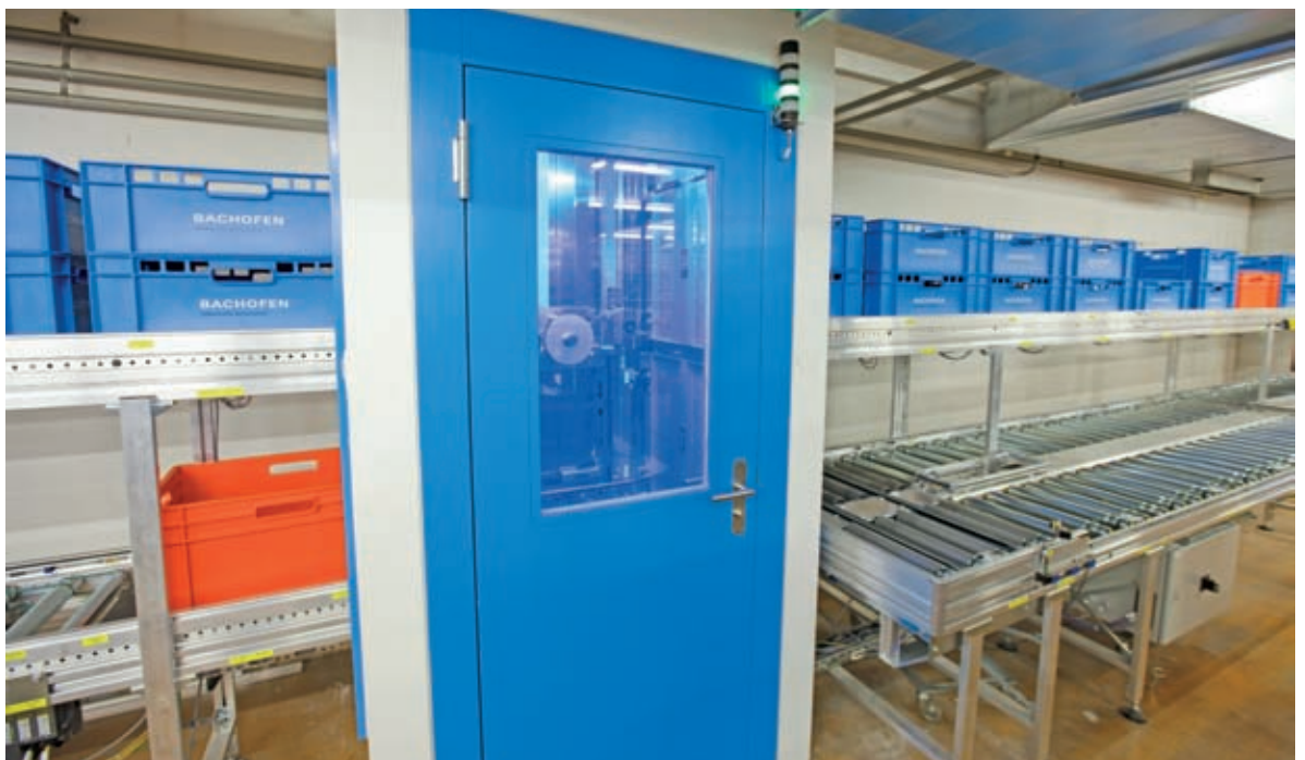
In front of the service lift, a read/write head reads the destination data from the tag at the bottom of the box
