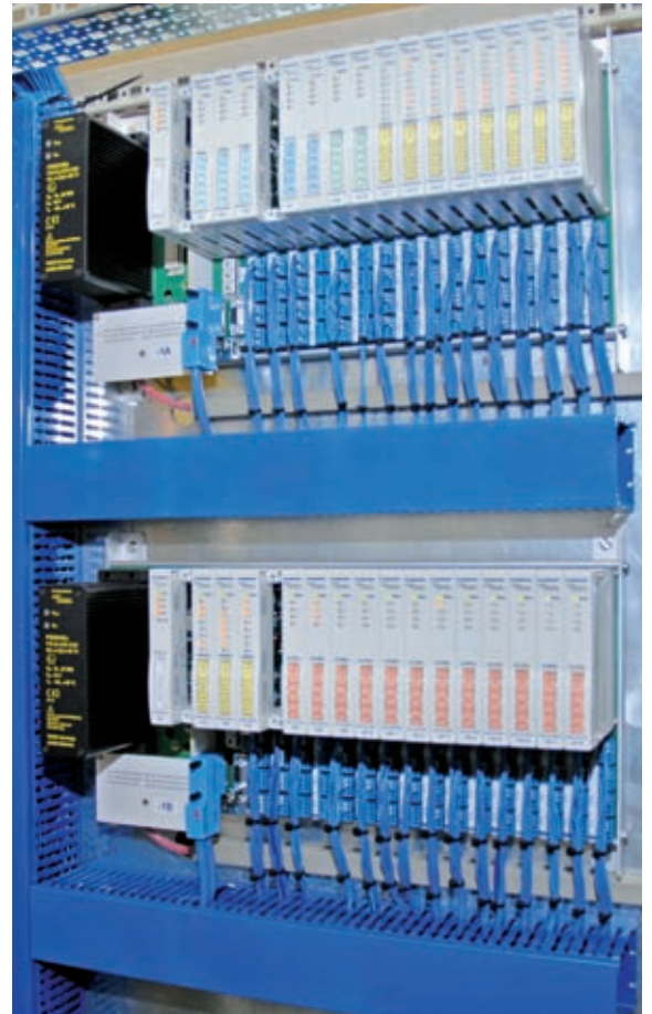
In only one weekend, EAB Automation installed the new excom systems into the 19" racks
