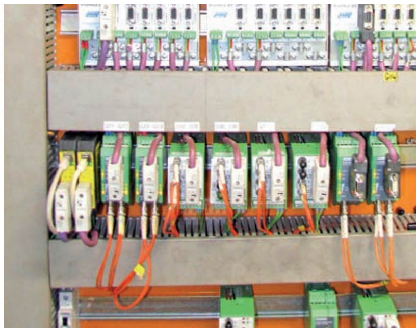
If the PB-XEPI is configured as a listener, the diagnose-tool is able to monitor the whole network without an own Profibus address
