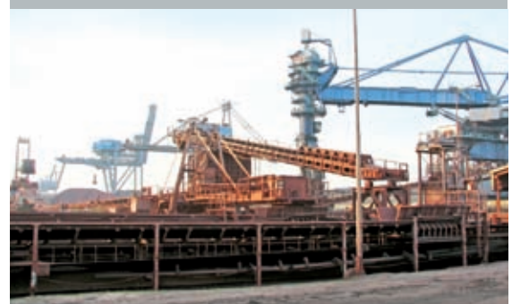
With the PB-XEPI, Ertsoverslagbedrijf C.V. in Rotterdam is able to identify disturbances of the Profibus-net centrally via web browser Page 38
