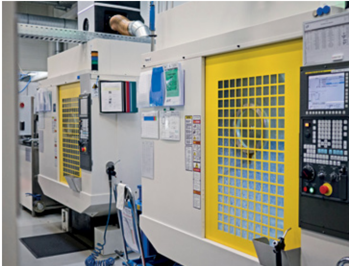
Communication with the KSS units of the four machines is implemented via Profinet
