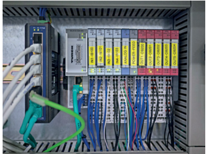
The central BL20 I/O station is located on the central lubrication plant and forwards all signals via Profinet to the TX513 HMI
